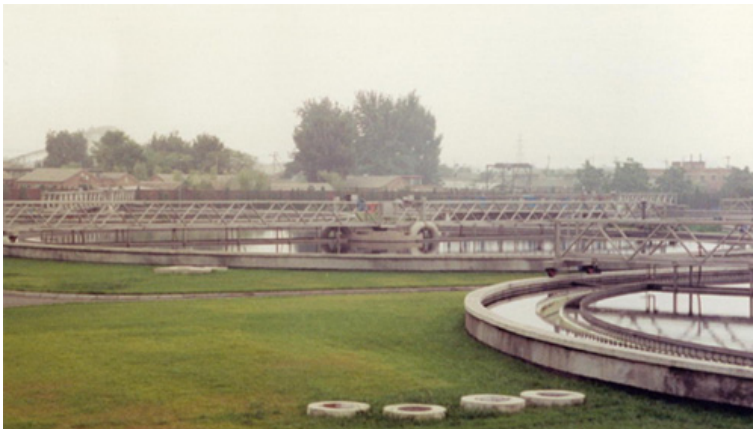
Appendix A.4 Tank at the Gaobeidian plant (studied in Chapter 3) Source: Beijing Water Authority
