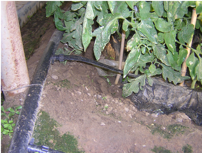
Appendix B.5 The pipes transferring collected rainwater from storage tank to plants
