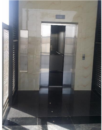
Photograph 23: Electric lift at Idu station Abuja
