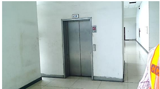
Photograph 24: Electric lift at National theatre station Lagos
