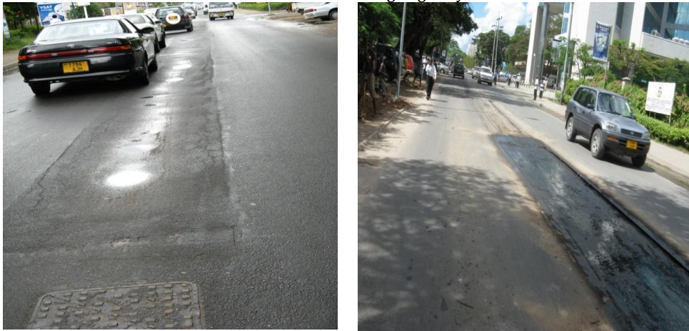
Figure 4.14 Road surface failures along Bagamoyo Road
