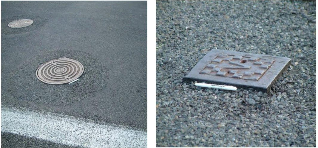
Figure 5.26 20 mm cover above carriageway in wheel path
