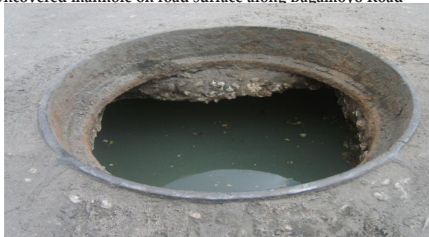
Figure 5.25 Uncovered manhole on road surface along Bagamoyo Road
