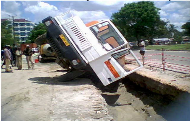
Figure 5.23 A vehicle accident in an unprotected excavation in study area
