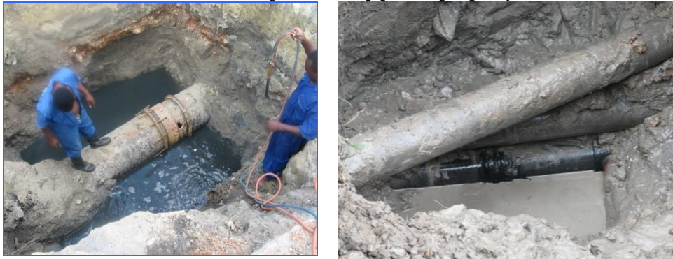
Figure 4.6 Condition of underground water pipes along Bagamoyo Road
