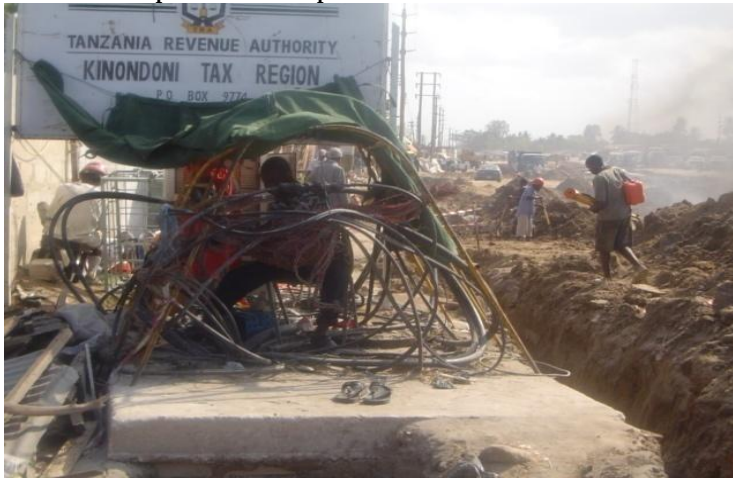
Figure 4.11 Operations of telephone cables in the road corridors
