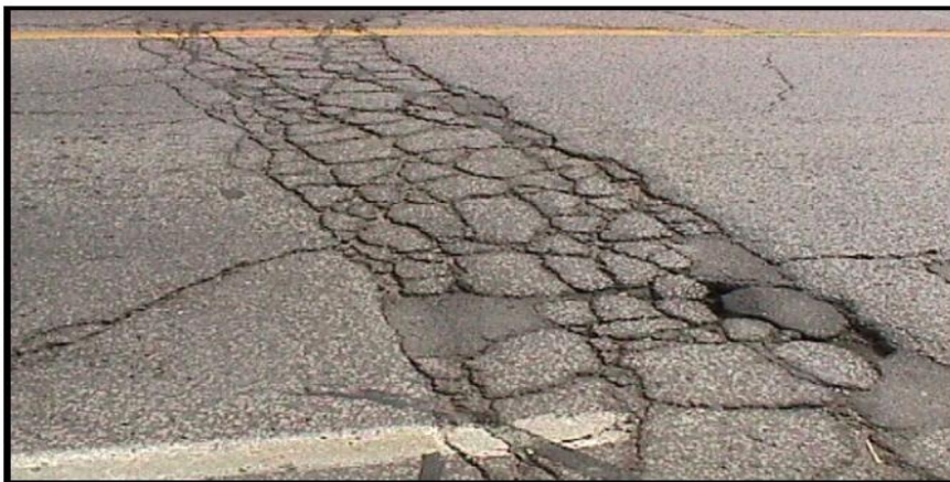
Figure 2.14 Reflective cracking from trench reinstatement
