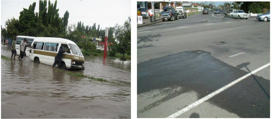
Figure 5.22 Water layer on road surface due to water pipes defects
