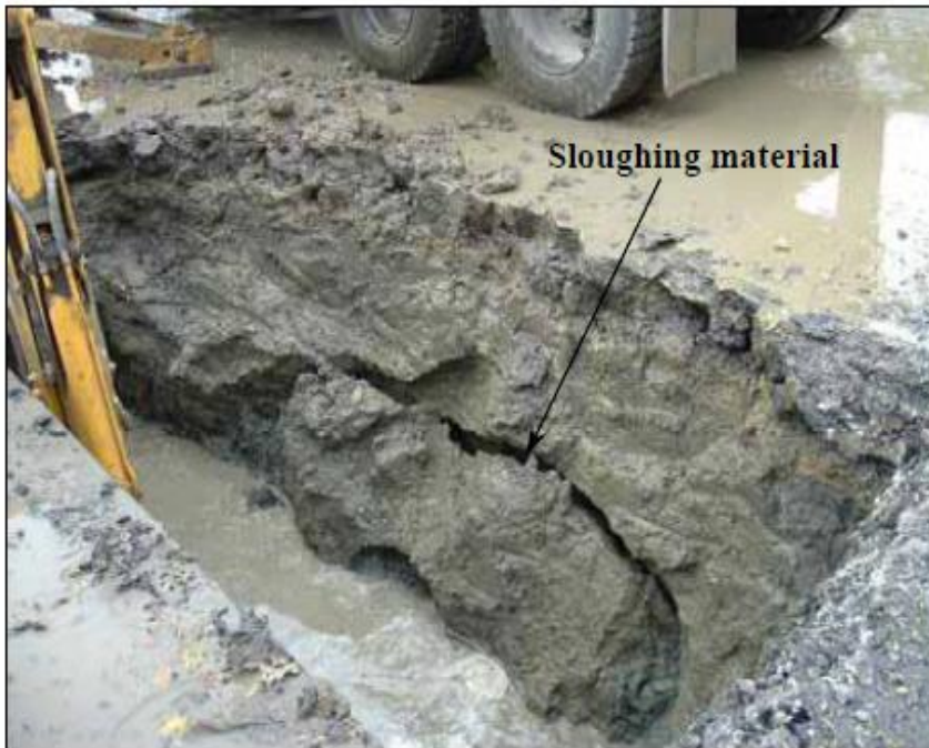
Figure 2.15 Material sloughing off edges of trench
